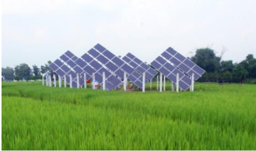
Solar Irrigation Pump
